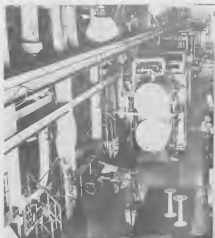
MODERN TURBO-generators , such as the one in the foreground of this No. 1 Powerhouse interior view, cost more than one half million United States dollars each. They convert steam power into electrical power.
